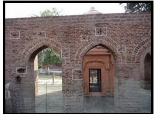
A building showing evidence of the damage caused by the bullets
